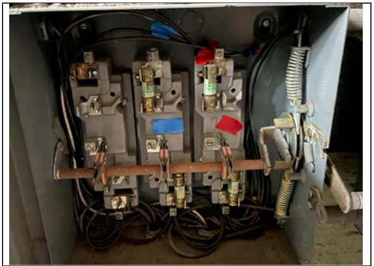
74. View of generator switch
