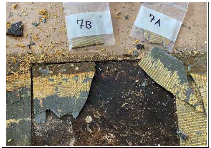
8. View of tan carpet mastic
