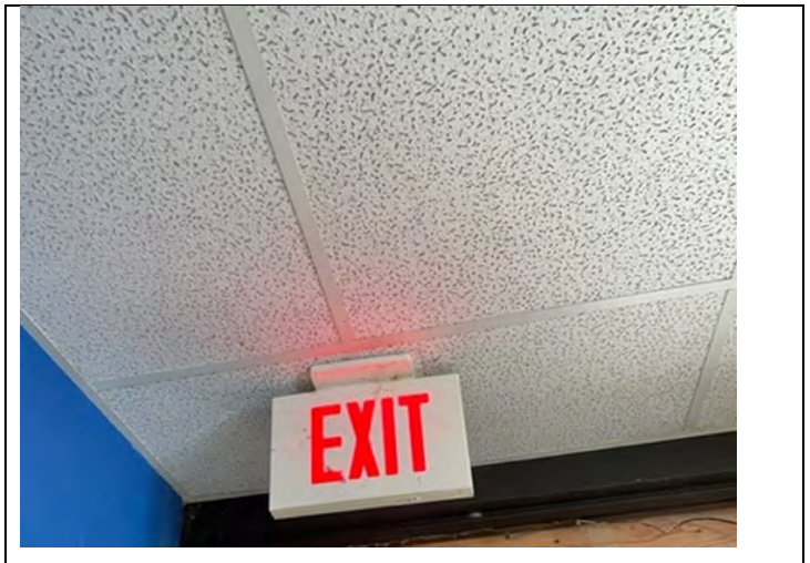
76. View of exit sign
