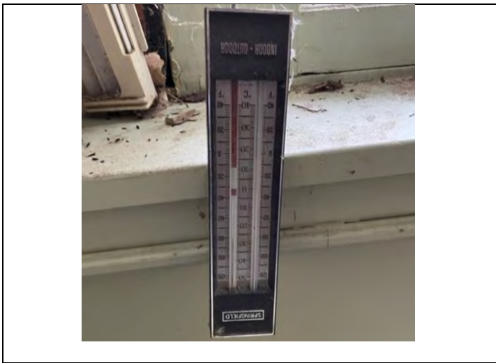
73. View of air conditioner thermometer
