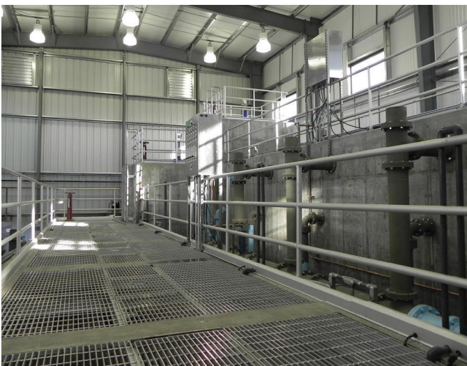
A Blue PRO installation in Grangeville, Idaho for 0.05 mg/L phosphorus with a chemical dose of only 10 mg/L of Fe.
